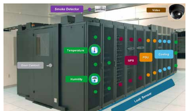
Monitoring and management of Data Center sensors
